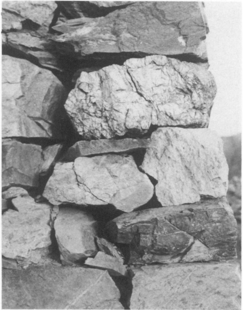
2. Careful stacking of the stones produced a square tower with a relatively smooth exterior (p. 181)
